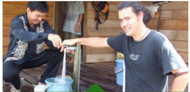
Water pipes and Mini-Hydro Dam for water
