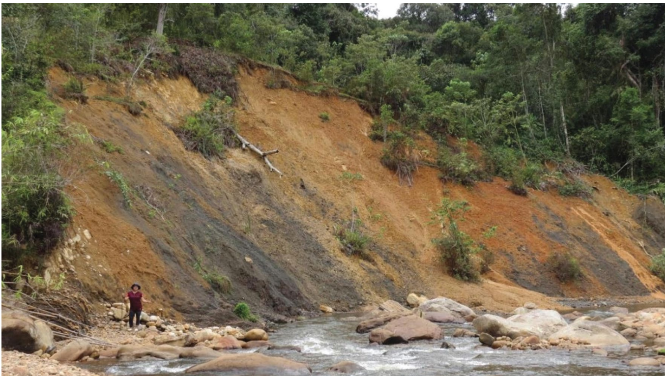
Close up pix of the erosion and landslide at the slope next to the river.
